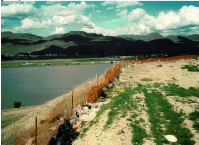
Mission Flats Landfill in Kamloops is unlined and built close to the Thompson River.
